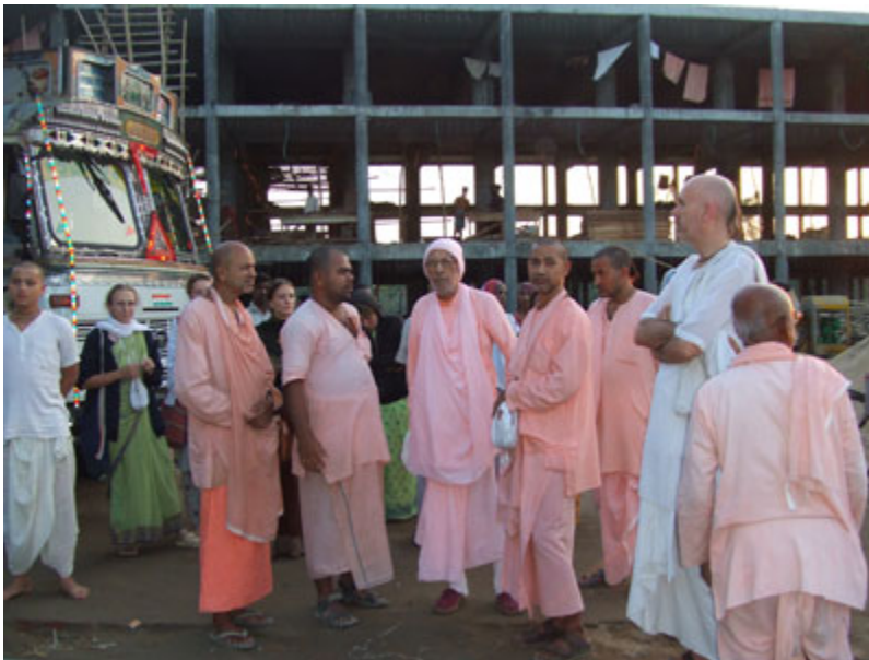
Looking at the ongoing construction of Sri Kesavaji Gaudiya Math in Navadvipa.
